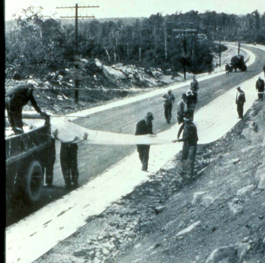
Surfacing soft shoulders with cloth-reinforced asphalt in Rhode Island. The cotton strips are being laid out to the toe of the slope to prevent erosion.
