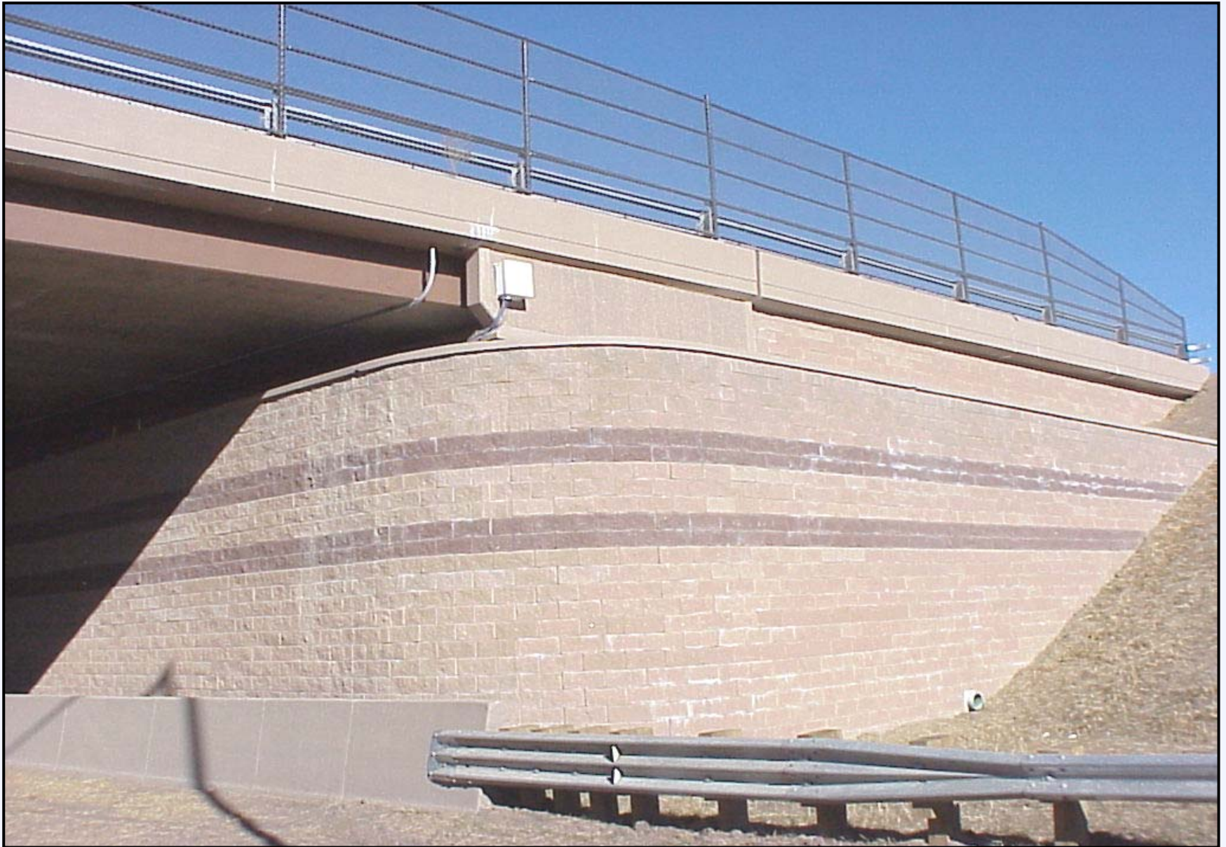
Founders Meadows Geosynthetic-reinforced Abutment (I-25, Exit 184)
